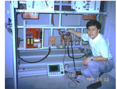
直流雜散電流檢測 DC traction system stray current Measurement and analysis
